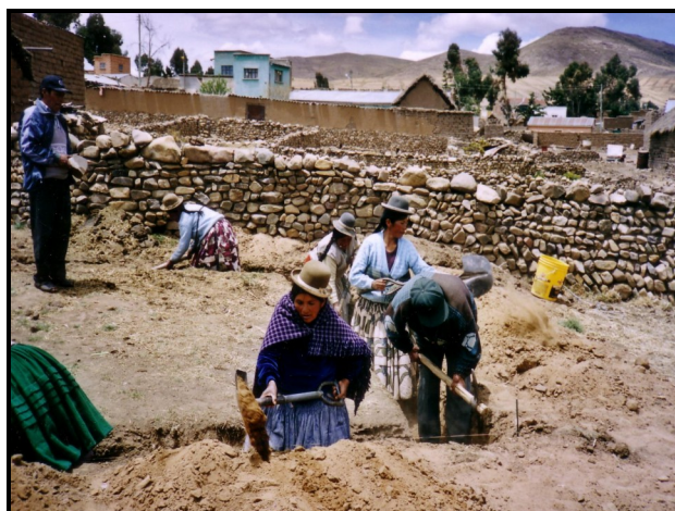
Community members may lay over two miles of piping to bring water to every house.
